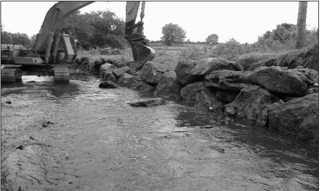
Bank restoration works underway on the Mad River, a tributary of the Moy
